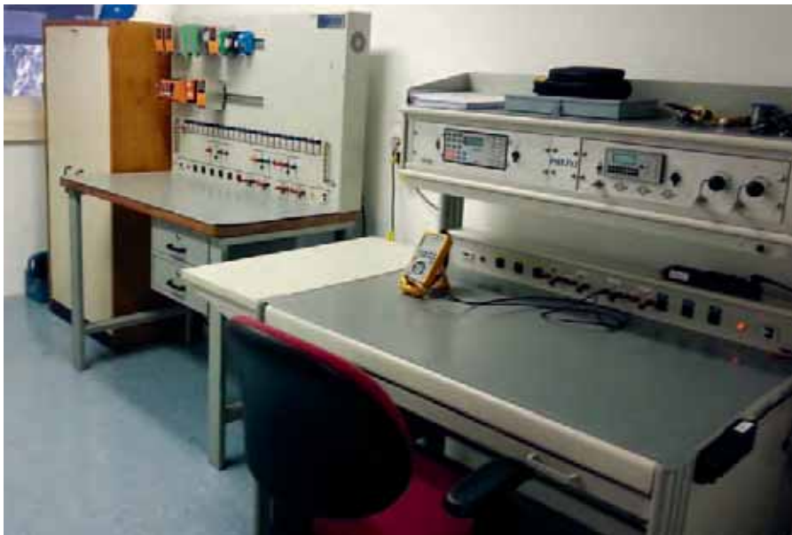
Test benches for instrumentation, PLCs, and communication networks
