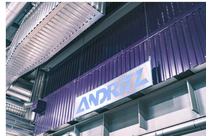
Helsingør Kraftvarmeværk specified colors of various equipment for the visual identification of different boiler parts.
