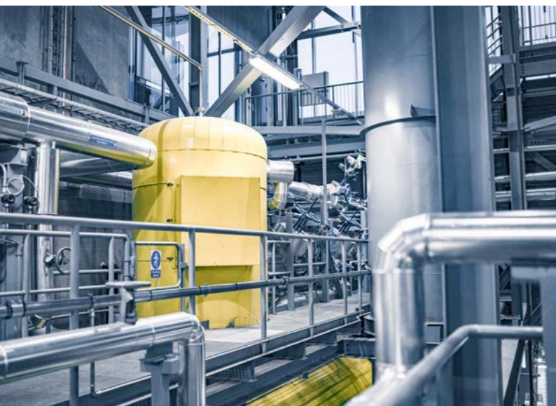
The boiler burns wood-based biomass, which consists of forest residues, bark, sawdust, and woodchips.
