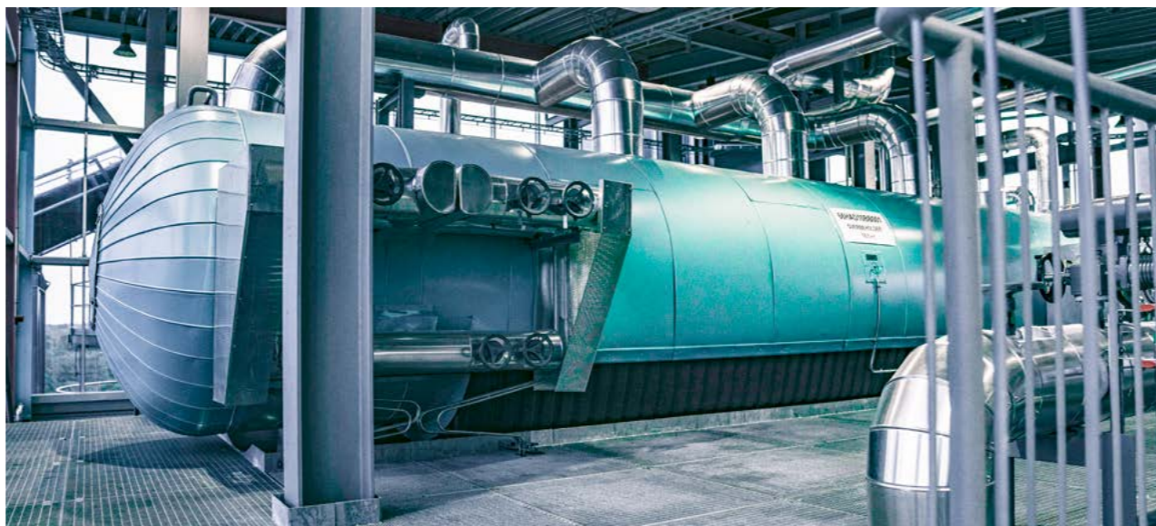
The steam temperature is around 500 °C with a steam pressure of 65 bar (a).
