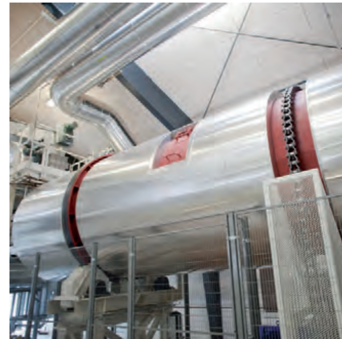
▲ The ANDRITZ rotary dryer at the Sdr. Stenderup plant dries biomass prior to entry into the torrefaction reactor.
