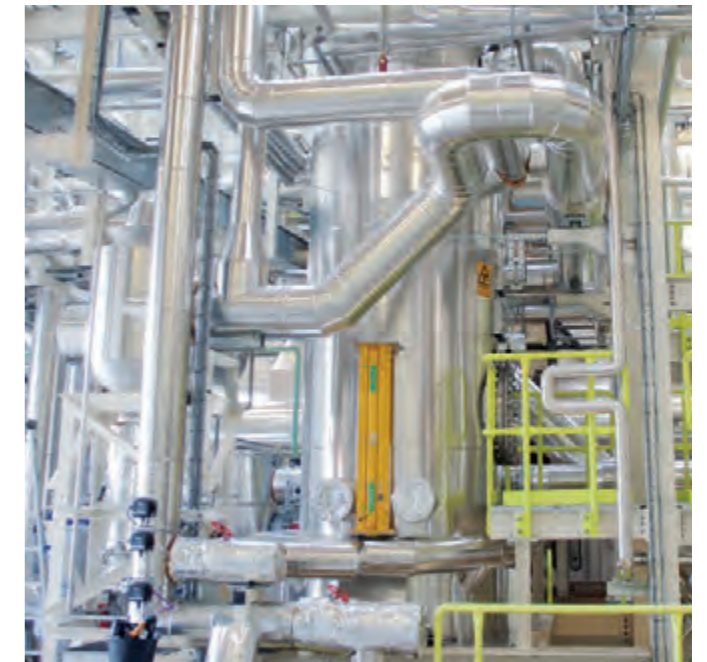
▲ Overview of the Sdr. Stenderup plant showing the ANDRITZ vertical pressurized torrefaction reactor.
