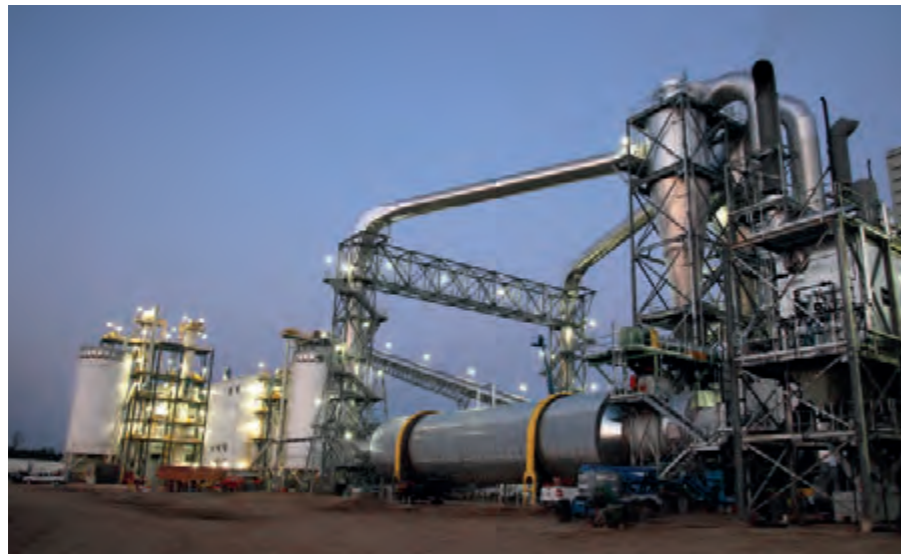
▲ It was only 14 months from the first turn of a shovel to production of the first pellet. This view shows the thermal driers and power boiler in the foreground (right) and the pellet plant in the background.
