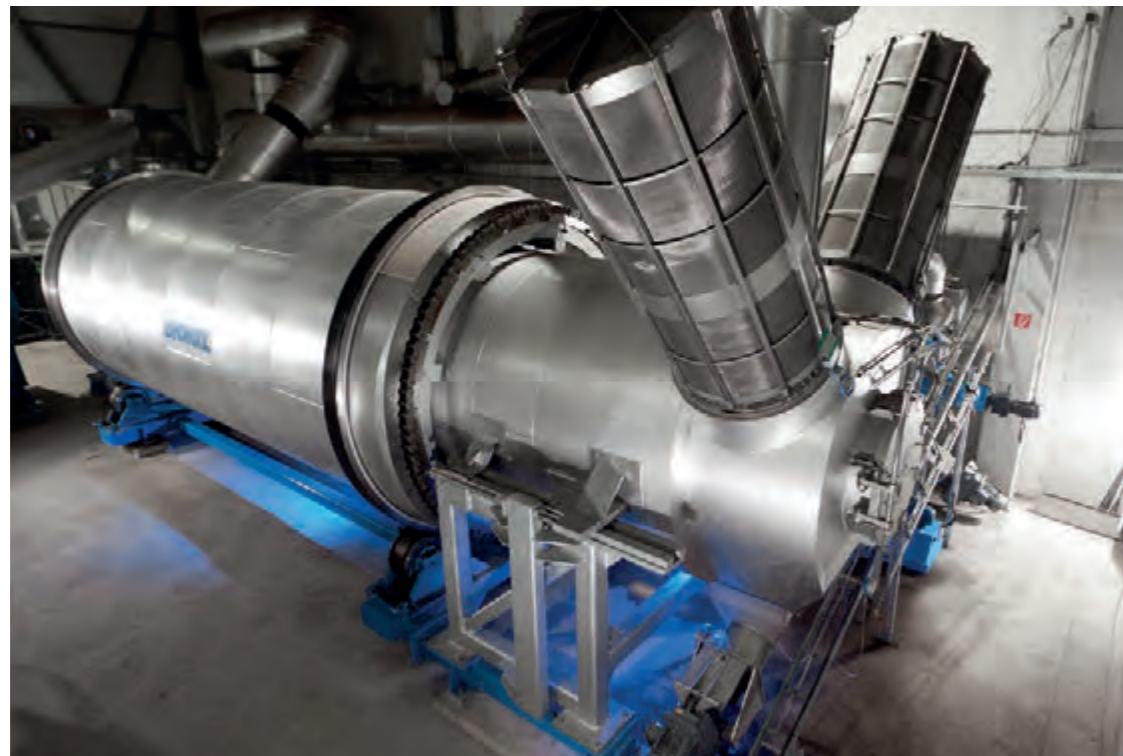
Torrefaction reactor at the ACB pilot plant in Frohnleiten, Austria. ▶
